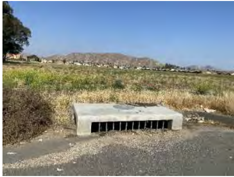
Photo 17: From Indian Street looking east towards an existing drainage inlet along the western boundary of the Project Site.
