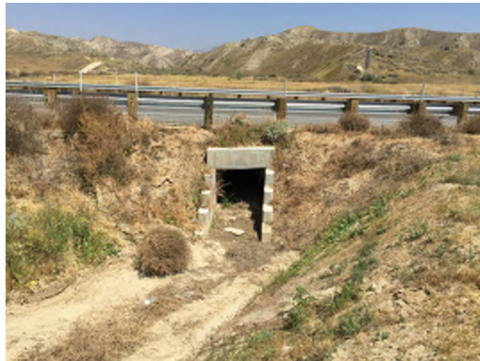
13. View of Drainage Feature I and the concrete box culvert on the westerly side of Gilman Springs Road. Photograph taken (April 1, 2015)
