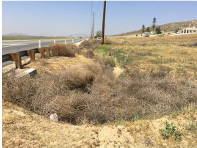
12. View of Drainage Feature I on the east side of Gilman Springs Road where it is filled with vegetative debris at the culvert entrance. Photograph taken (April 1, 2015)
