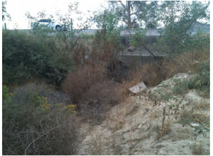
10. View of Drainage Feature G and its concrete culvert at SR-60. Photograph taken (October 7, 2013)
