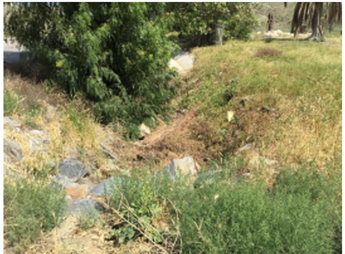
4. View of Drainage Feature H where it drains under Theodore Street to the west. This drainage is primarily a concrete lined v-ditch paralleling Ironwood Avenue. Photograph taken (April 1, 2015)
