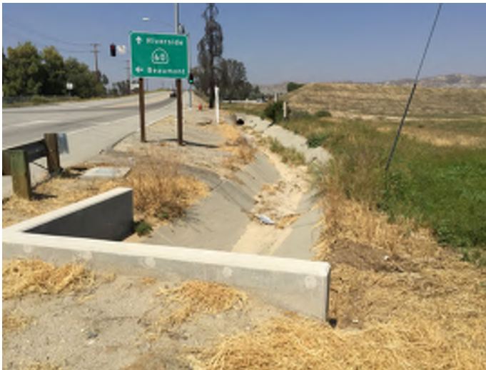
3. View of Drainage Feature B near the Redlands Boulevard on-ramp where it is a trapezoidal concrete lined channel. Photograph taken (April 1, 2015)
