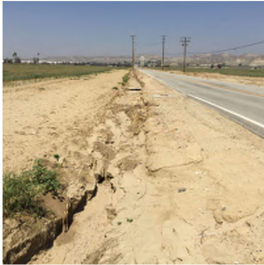
9. View of Drainage Feature F northwest of the intersection of World Logistics Center Parkway and Alessandro Boulevard. Photograph taken (April 1, 2015)
