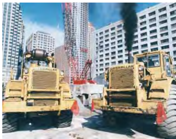
Retrofits are effective in reducing particle emissions from heavy equipment. The tractor on the left is retrofitted with a particle emissions control device.
