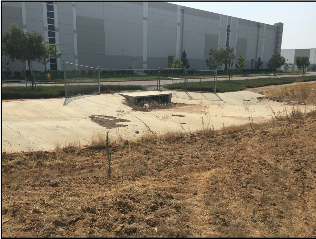
Plate 5.2–4: View of a storm drain found along the southern boundary of the subject property, facing south.
