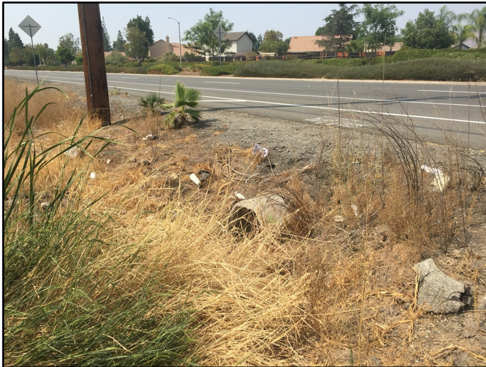
Plate 5.2–3: View of a concrete culvert designed to direct water under Alessandro Boulevard onto the subject property, facing north.
